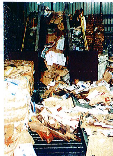
Infeed conveyor into a solid waste baling plant (USA)
